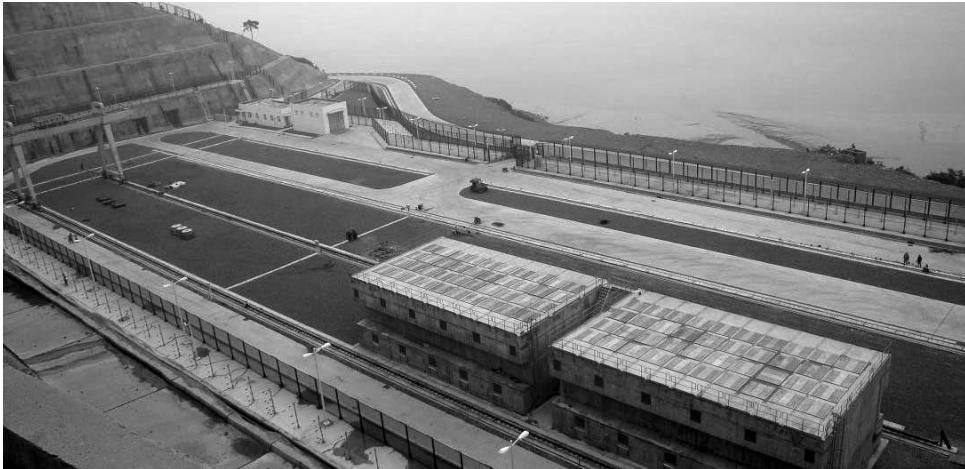
Figure 2.1. Macstor-400 Dry Cask Spent Fuel Storage at Qinshan III NPP. The black squares are vents for convective circulation of air. Source: Beijing Starbecs Engineering Management Co.
