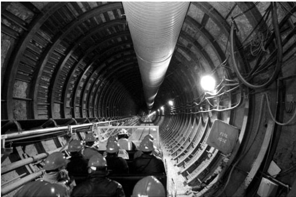
Figure 10.3: Workers carried in an open rail car enter the main tunnel under Yucca Mountain. The
