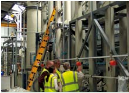
Commissioning activities on the cylinder washing and cut-up being built at Capenhurst.
