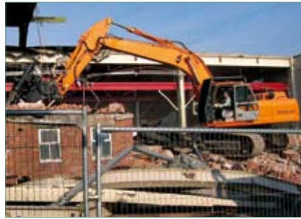
The continued safe demolition of buildings, which are redundant to the ongoing storage business within the first three years of the Lifetime Plan.
