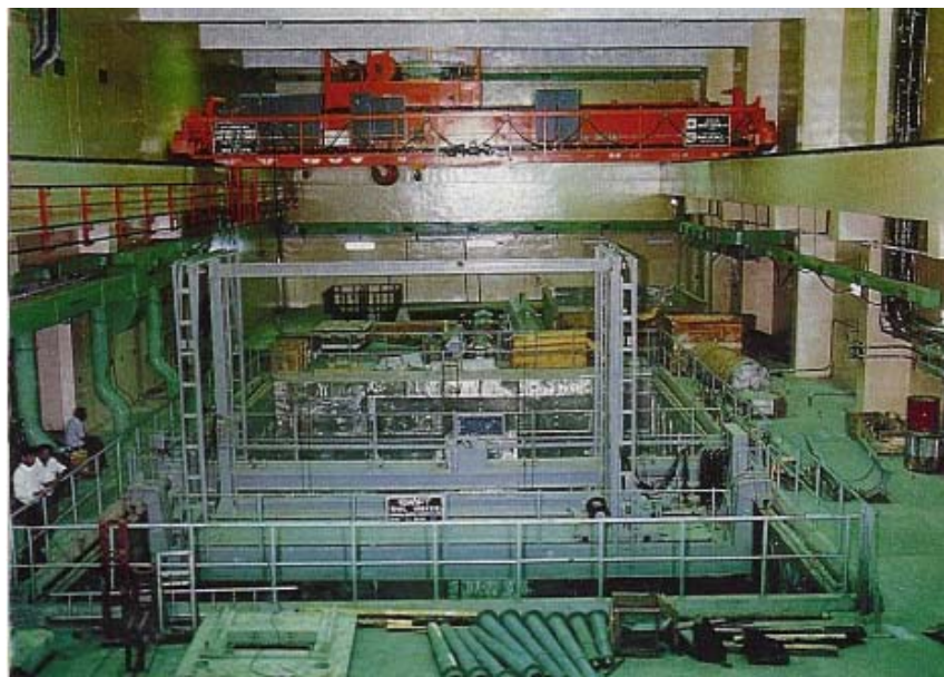
Figure 4. Spent fuel pool and fuel handling area, Kalpakkam reprocessing plant. 53
