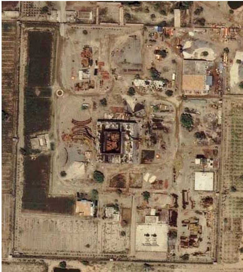
Figure 3. The reactor under construction at Khushab (12 August 2006; IKONOS satellite image courtesy of GeoEye).
