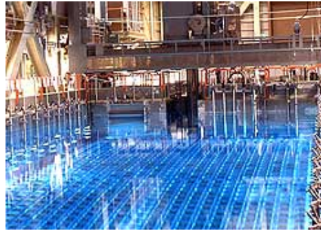
Figure 2.2. Spent-fuel storage pool at nuclear power plant 14
